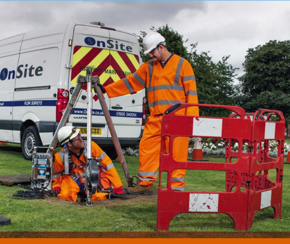
Above: Flow monitoring equipment measures the depth of flow and velocity in pipelines (Picture credit: OnSite)
